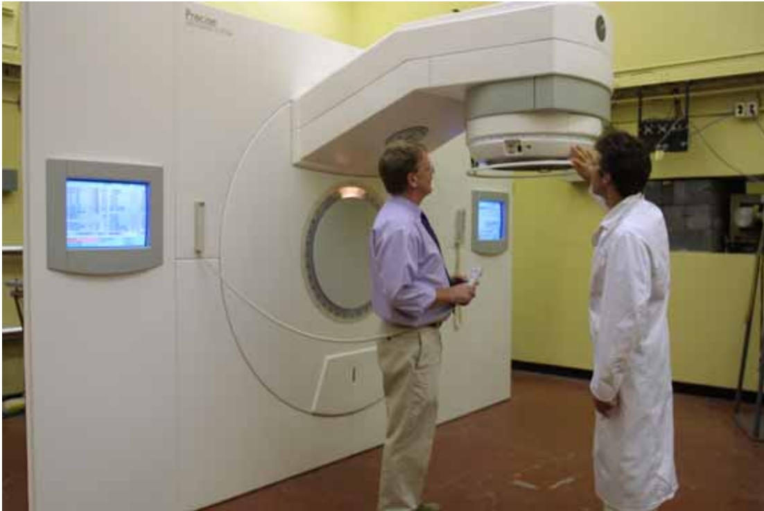
Figure 1. Completed installation of the Elekta Precise linac in the NRC accelerator hall.
